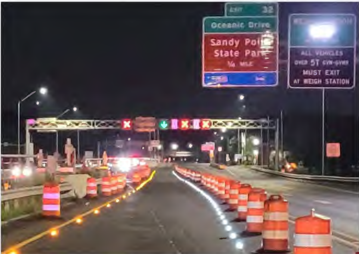
At the Chesapeake Bay Bridges LEDline® Helps Guidance at Their Rush Hour Contraflow Control.
