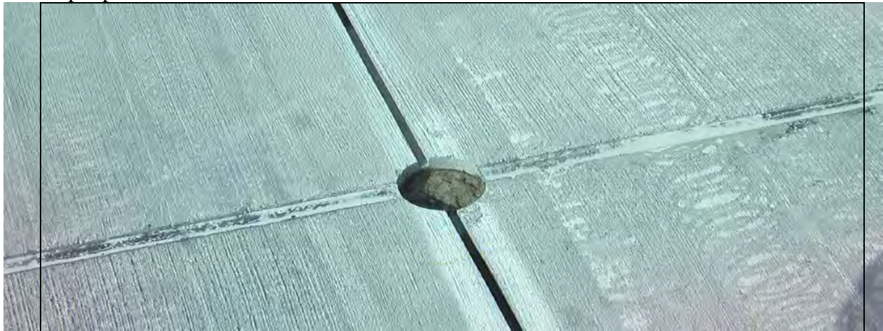
Fig. 1. 100mm (4") diameter cut hole across an expansion joint to allow for a wire a service loop top move with the different slabs.
